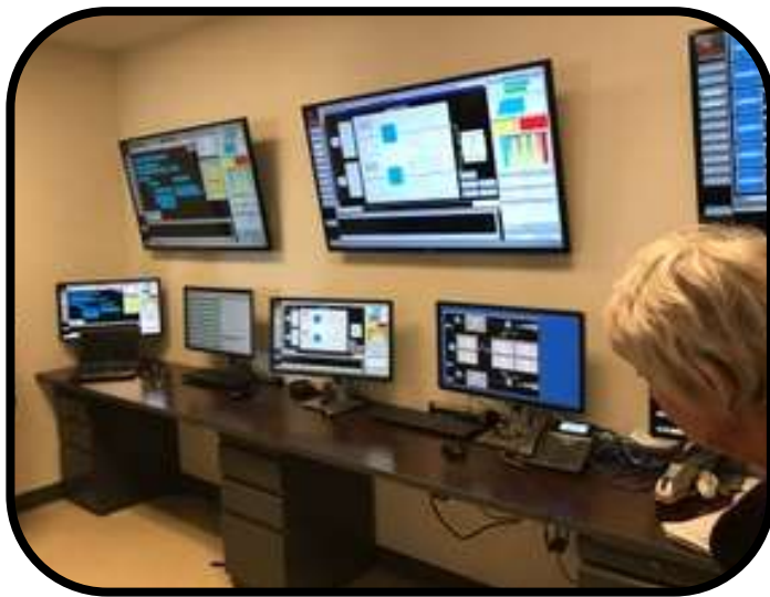
Figure 3 Solar Control Room
