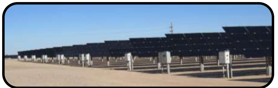
Figure 5 Tenaska Solar Energy Farm
